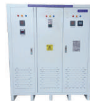
Isolation Transformer (K-13)
